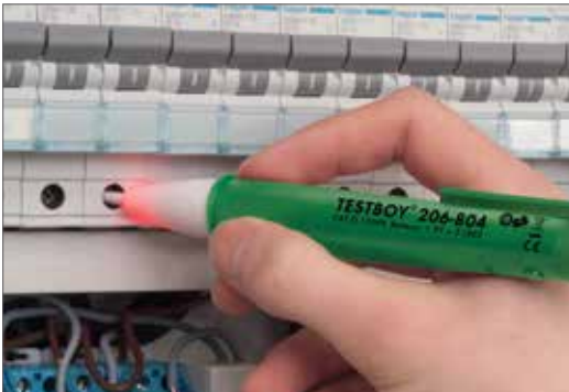
Testboy illuminates with voltage present
